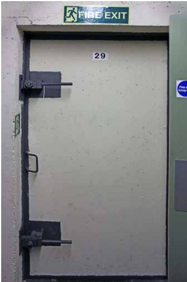
Interior view of emergency escape at upper level. One of the many reinforced concrete blast doors surviving in fantastic condition
